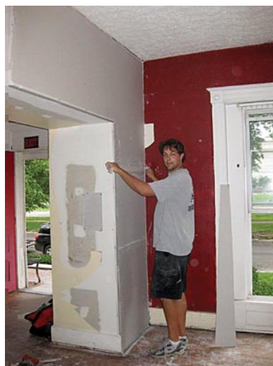
Clockwise from top: Alumni attend a Christmas party at the house. Landscaping will get tidied up even more in the next phase. Drywall is installed and sanded. The new chapter room pulls it all together.
